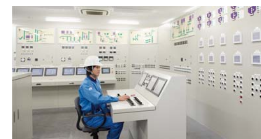
Centralized control room
